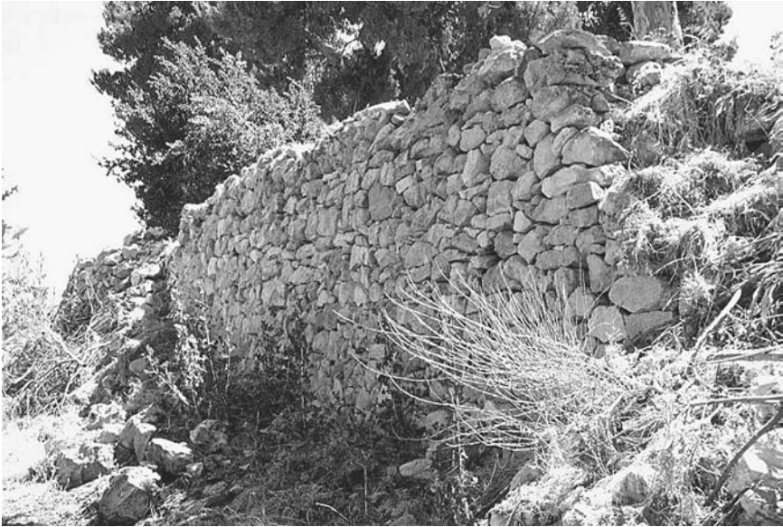
Figure 5. Retaining wall of the platform on the summit of Ras et-Tabuneh at el-Bira (photo by Michael Luddeni).
